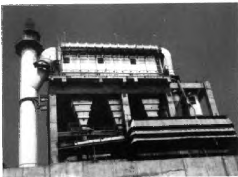
ESP for Cement Mill
